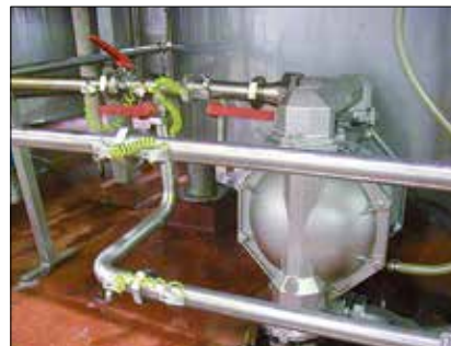
3" sanitary pump used to transfer cosmetic basis for shampoos
